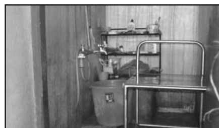
A simple hose attached to the tap.
